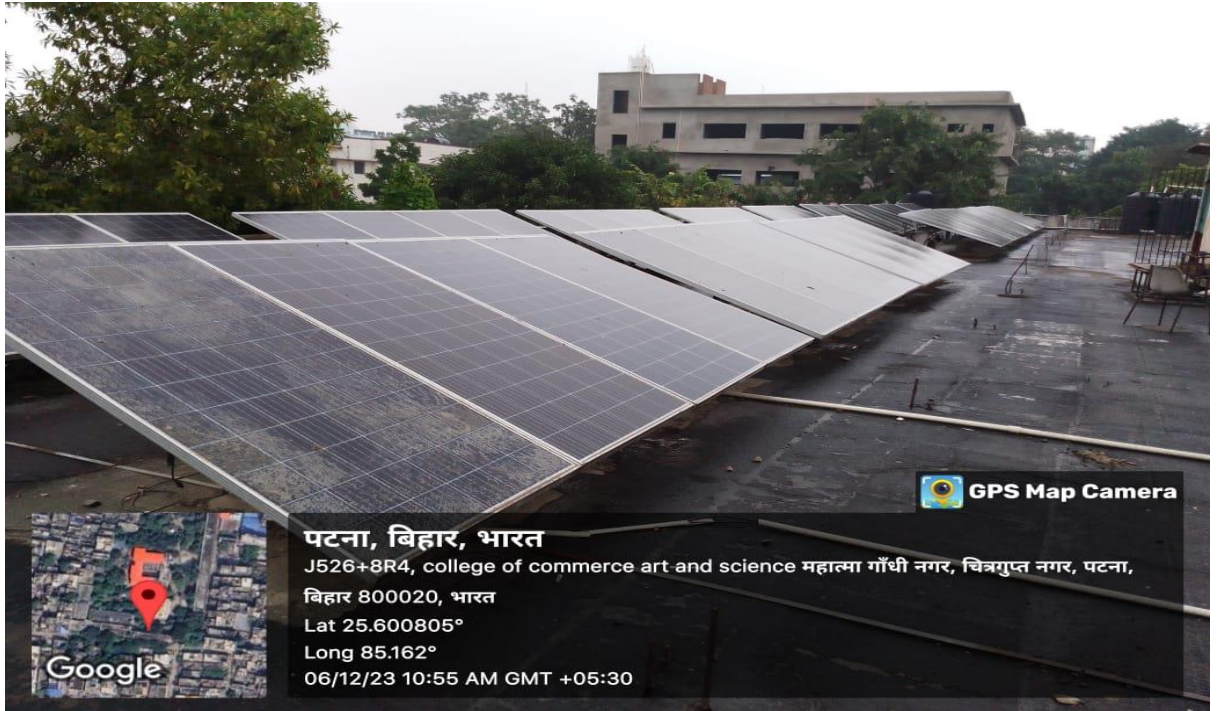
Fig.:Solar Panels installed in the campus
